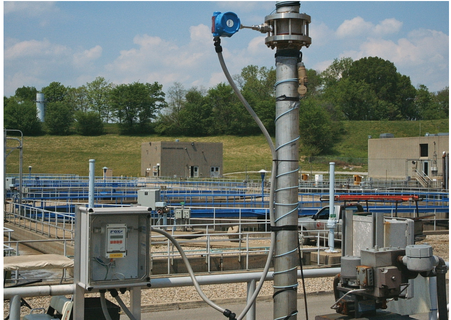
Here a thermal mass flowmeter is used for off-gas monitoring in a wastewater treatment facility. The instrument's low-flow measurement capability and data-logging software help operators diagnose upset issues to improve process control.
